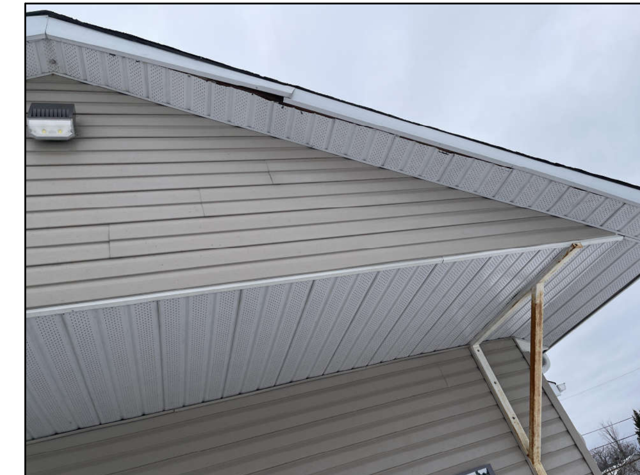
PHOTO - DAMAGED SOFFIT AND FASCIA (TO BE REPAIRED)
